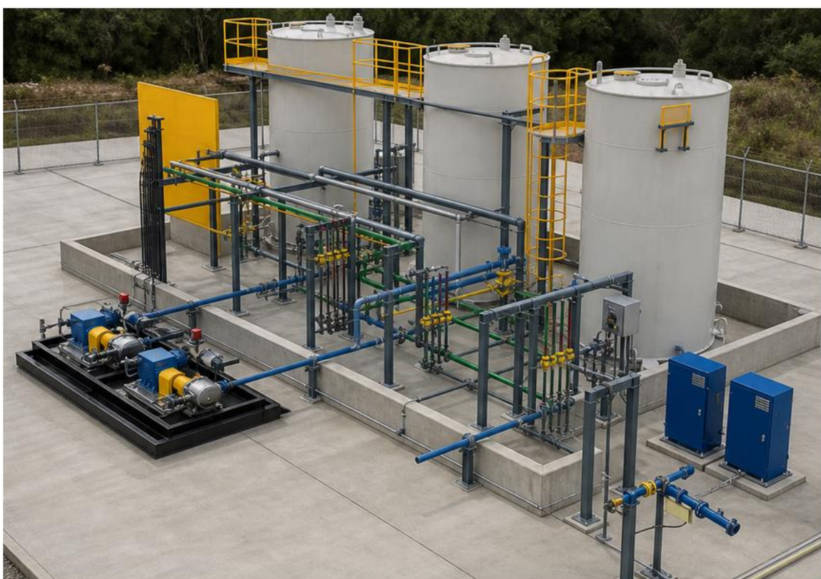
Case 1 - Tank farm / process piping
